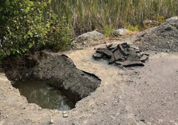
Road damage at Crystal Lake access site in the Panhandle Region
